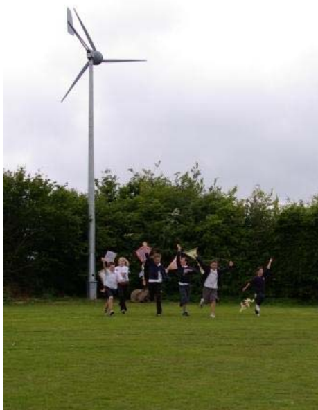
Figure 5: An Iskra AT5 - 1 installed.
