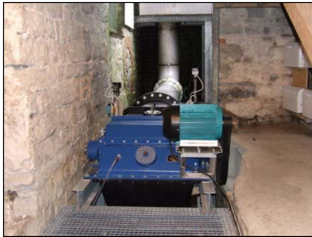
Figure 16 – Typical Ossberger Crossflow turbine installation. (Town Mill, Lyme Regis, Devon).
