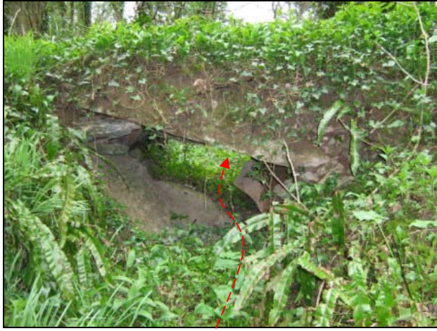
Figure 12 – Impediment to flow – rock lying across leat.
