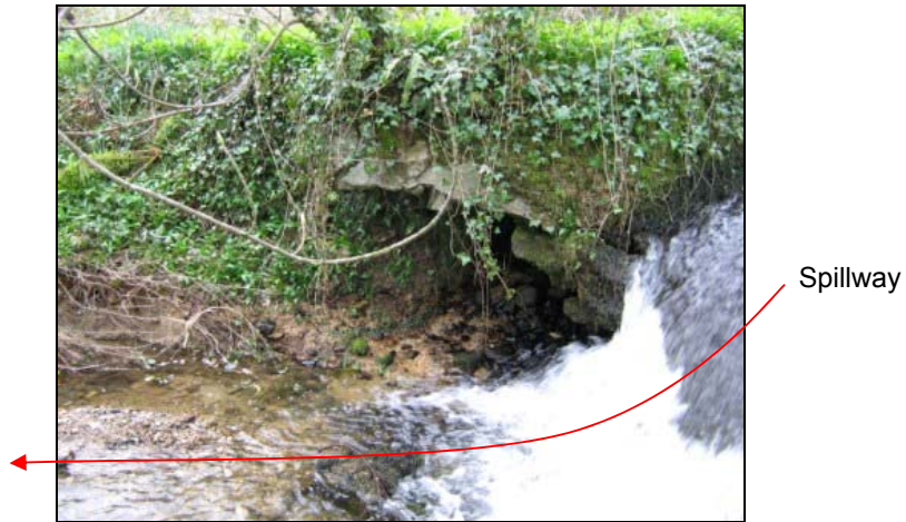
Figure 9 – Stone structure adjacent to spillway. This may have been a channel which allowed the leat to be drained while the sluice remained closed
