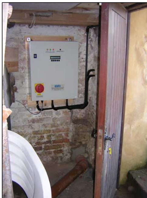
Figure 24 – G83 grid connection unit / hydro system controller.
